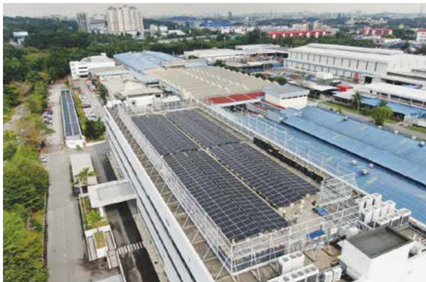
SA1 Plant Solar Panel System
